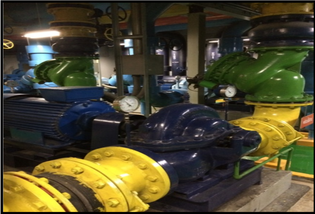
រូបទី ៣.5 chilled water pump 5
