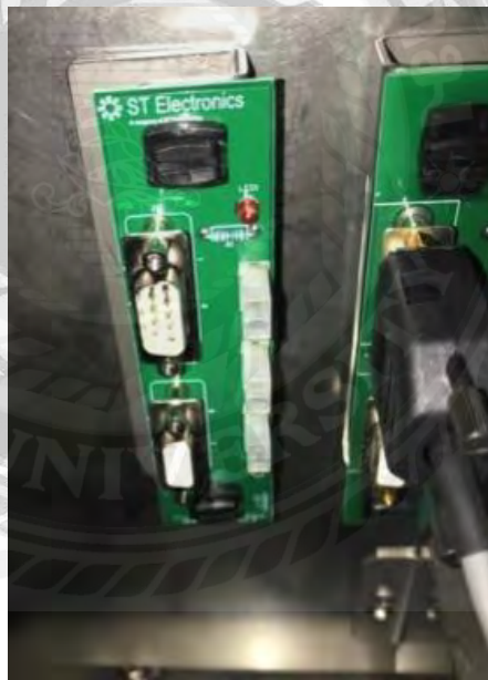
Figure 5-29 Fire Alarm Interface Board
