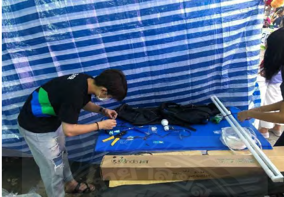
Figure 19: Set up lighting system in boost at Samut Prakan
