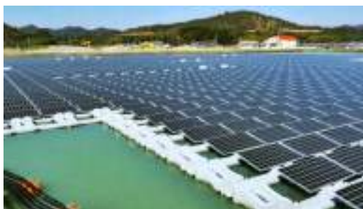
2.20 Floating Solar Cells
