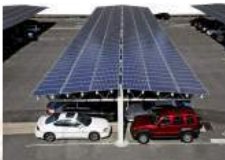
2.19 Fixed Solar Cells System
