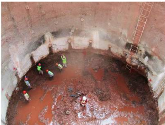
Fig.9 Excavation at Elevation 357-358 Fault material, (Date picture22/11/2017)
